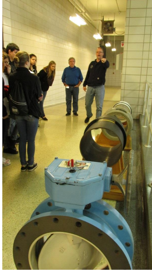
Weed pointing out the different types of valves DWC utilizes in the field
