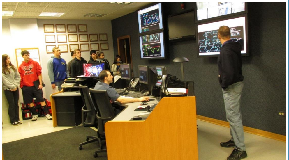
Mike Weed showing the students DWC's SCADA system in the control room
